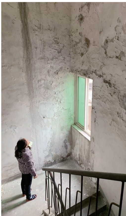
▲湘苑小区4栋2单元的楼顶渗水严重,墙面严重受损
