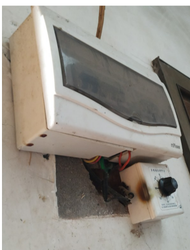
▲电表有被烧的痕迹
